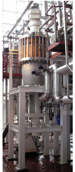
Wash Column Unit
