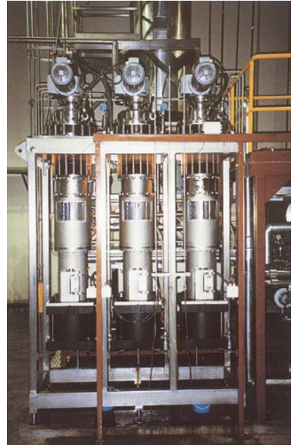
Wash Column Unit
