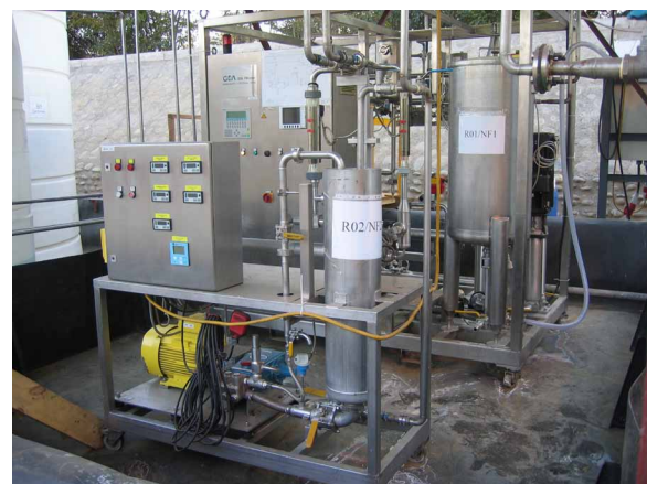
Pilot plant: RO unit section
