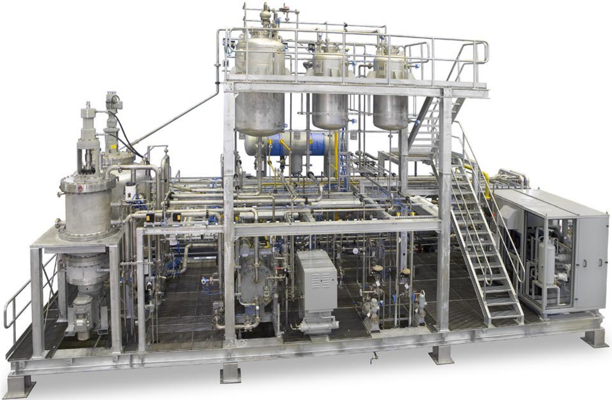
Skid mounted melt crystallization plant for purification of enantiomers
