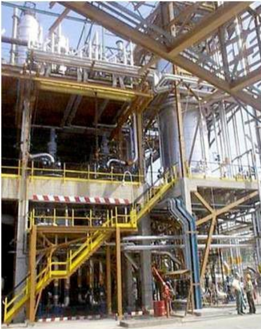
Melt crystallization plant for purification of paraxylene
