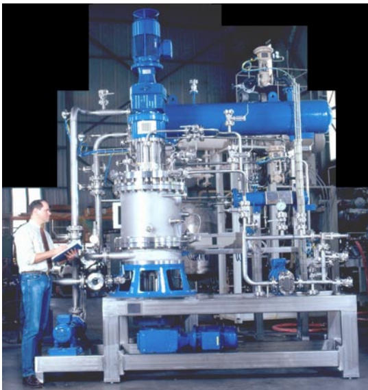
Industrial screw type GEA Messo PT Purifier. The crystal bed fills the cylinder between the main cylinder flanges near the center of the photo.
